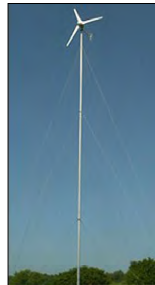
Figura 3: Torre con riendas (Wind Turbine Towers)
